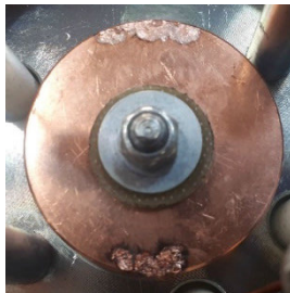
FIGURE 7. After a couple of attempts at switching the motor start.
