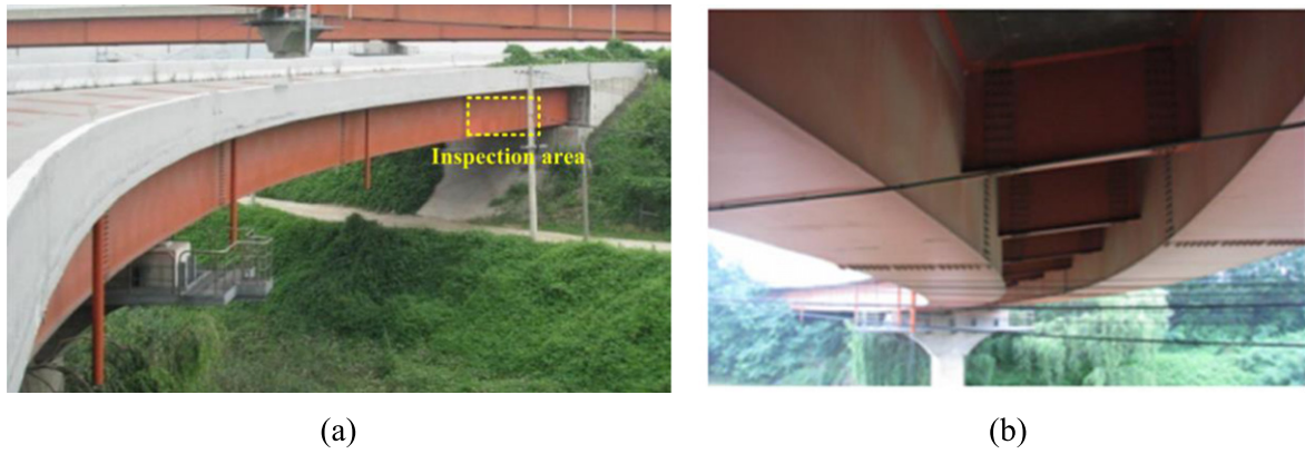
Figure 5. Decommissioned Ramp-G Bridge in Goyang, Gyunggi, Korea: (a) overview and (b) bottom view. Curved 90 m-long Ramp-G Bridge has two steel box girders.
