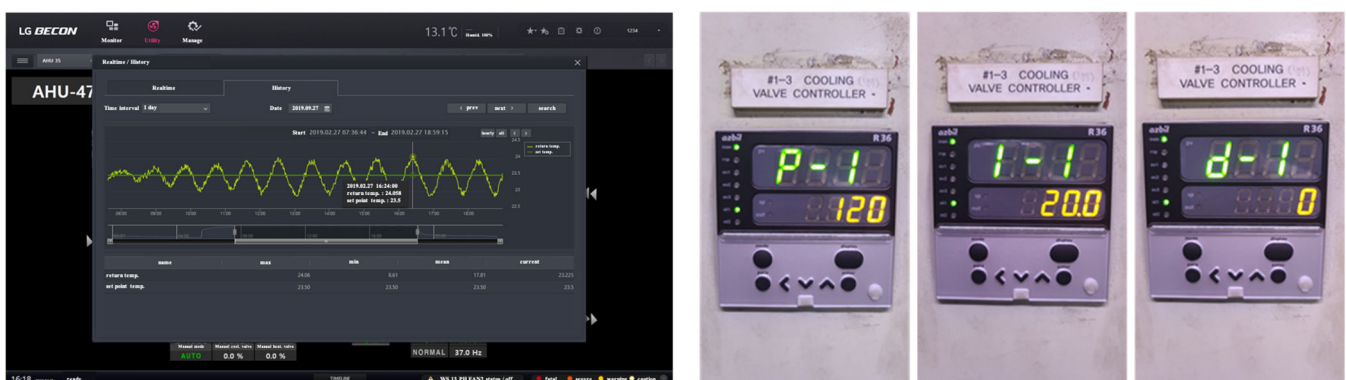
Figure 3. Building energy management system (BEMS) and cooling valve controller.
