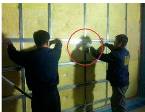
Figure 1. Resilient channel installation method (workers are fixing resilient channels to C-studs using screws).
