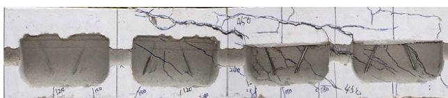
Fig. 10 Exposed lattes out of concrete
