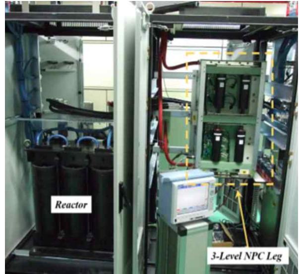
Fig. 13. 7MW(3,300V, 1500A) 3-level NPC converter test
