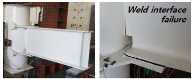
(a) Joint Failure
