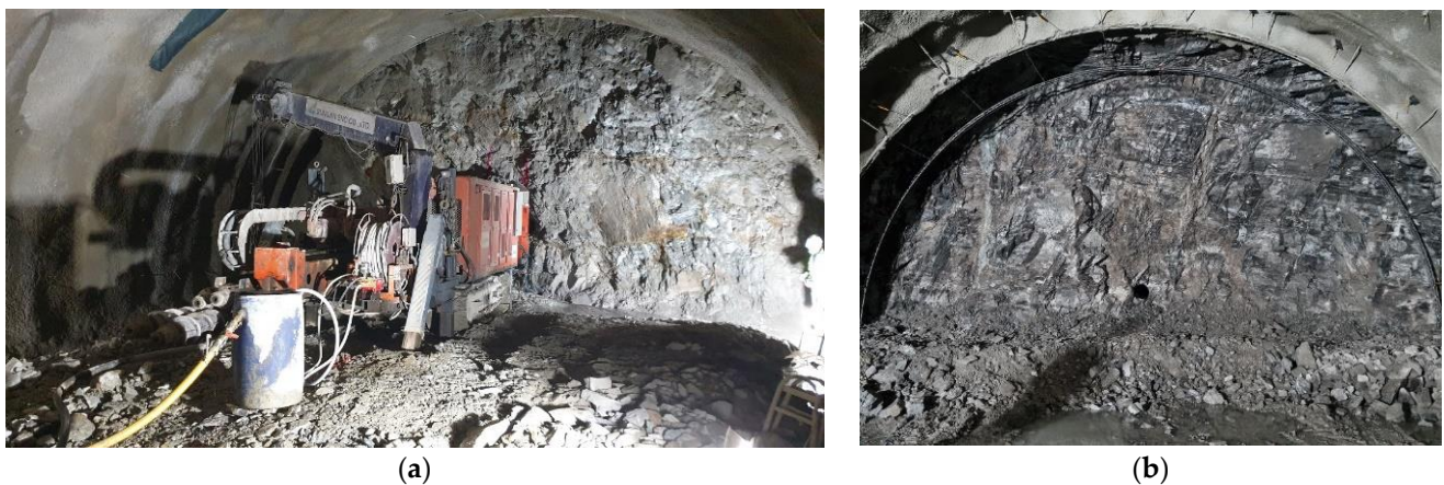
Figure 2. Images of field application of the LLB machine and a tunnel face with completed drilling. (a) Field application of the LLB machine; (b) tunnel face with completed drilling.
