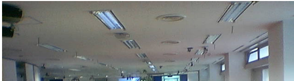
Fig. 2. Ceiling of the South Laboratory with installed sensors
