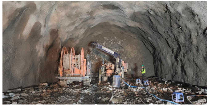
Figure 2. Photograph of field application of the LLB method at a tunnel construction site located in South Korea.
